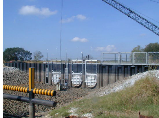
Controlled flap-gates help optimize water levels and salinity.
