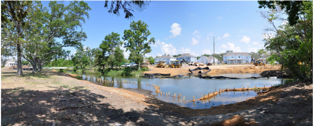
Post excavation of entire area, and bayou enhancement prior to installing wetland vegetation.
